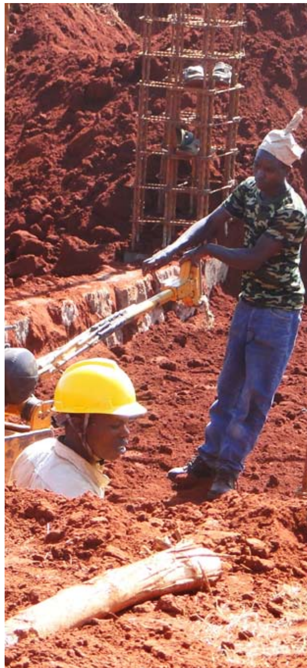
Construction workers lay the foundation for the upcoming APHRC office complex in Kitsuru, Nairobi.
