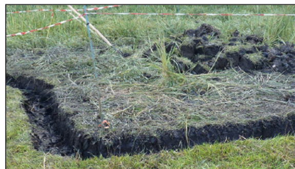
Action 2. The digging of small trenches near the Spartina alterniflora area to avoid its spread
